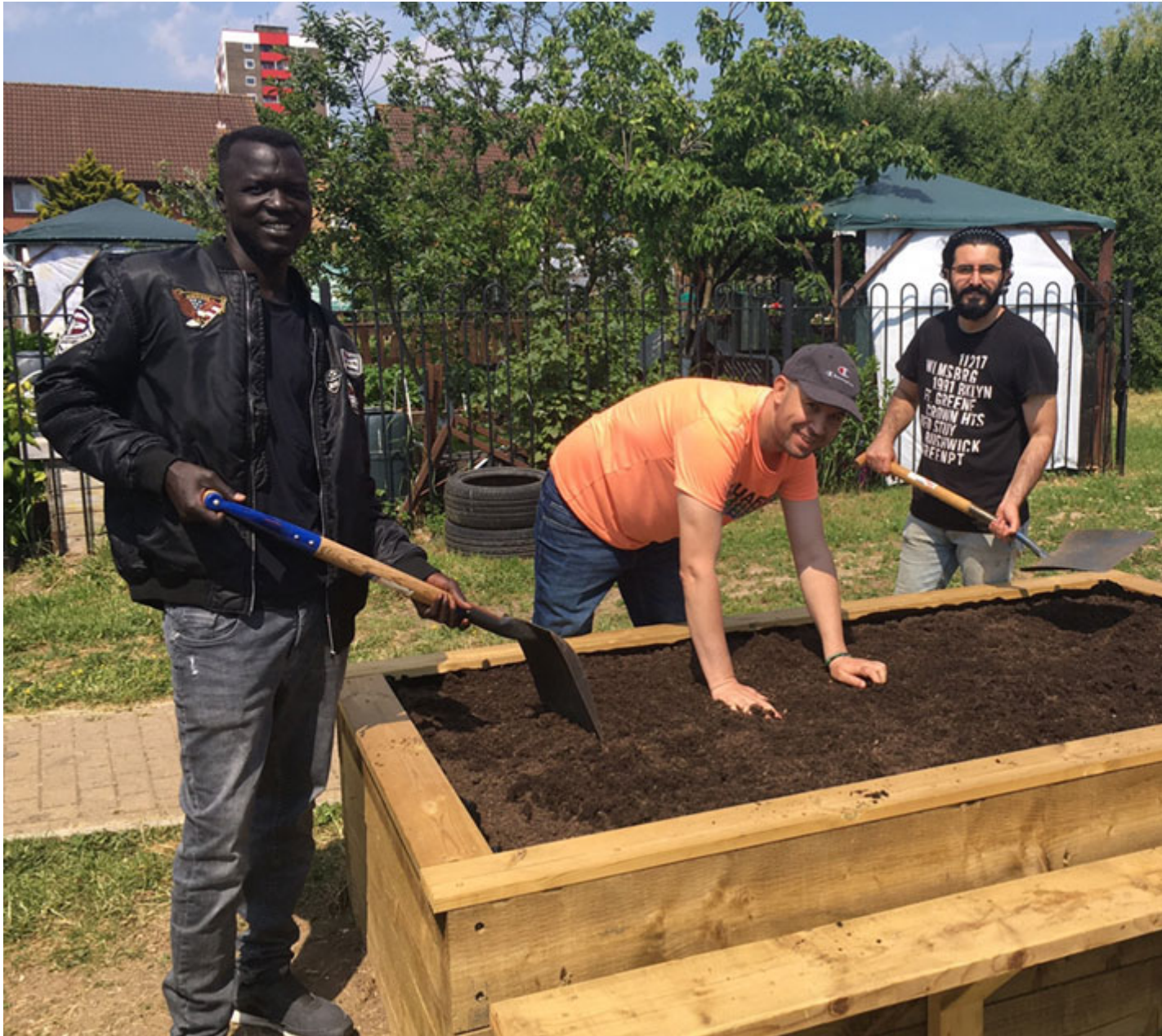
A raised garden bed constructed in Hull as part of Nextdoor Nature. Image: Andy-Steele.
