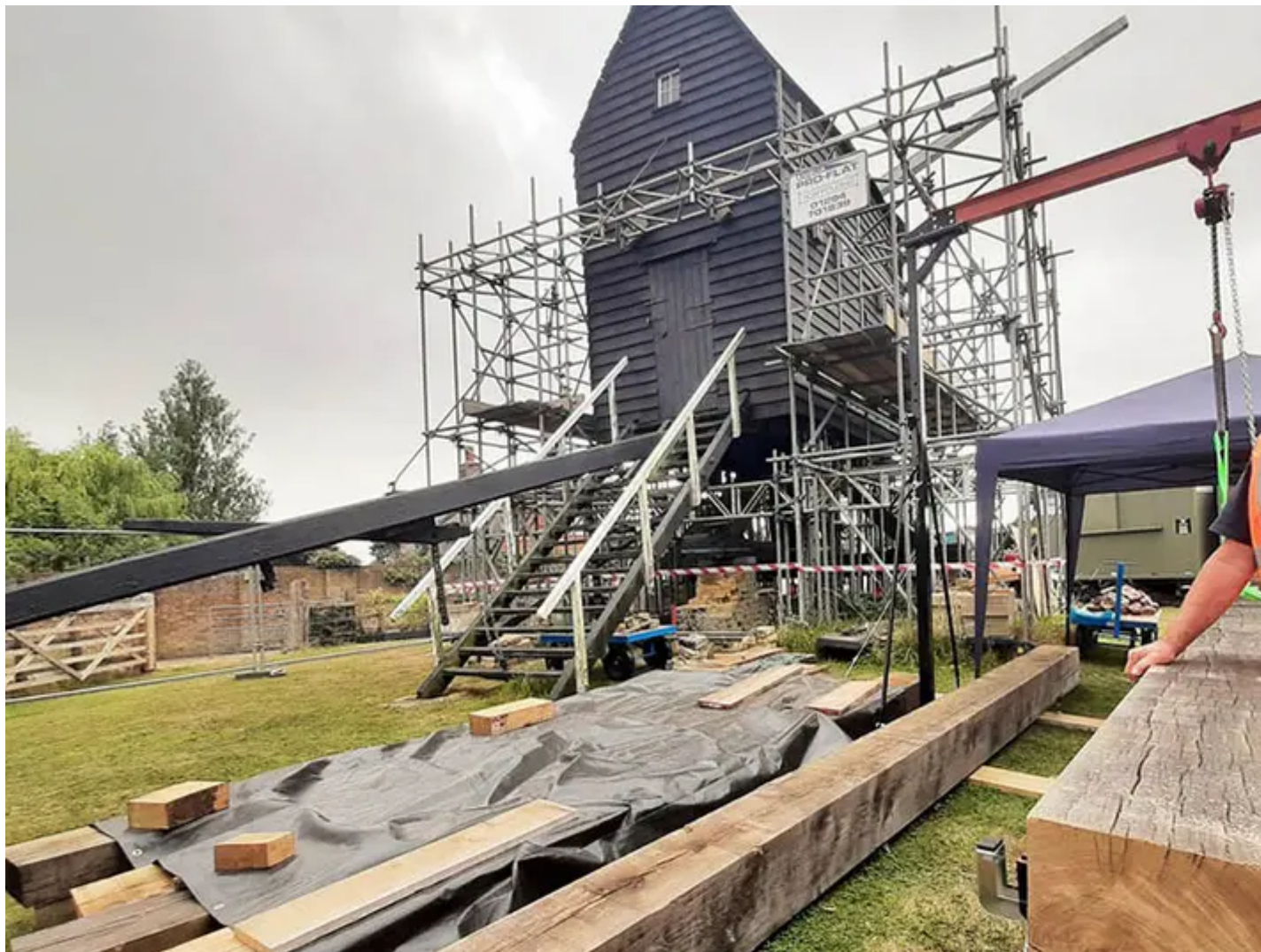
Scaffolding lifted the mill while the huge oak beams that support it were replaced.
