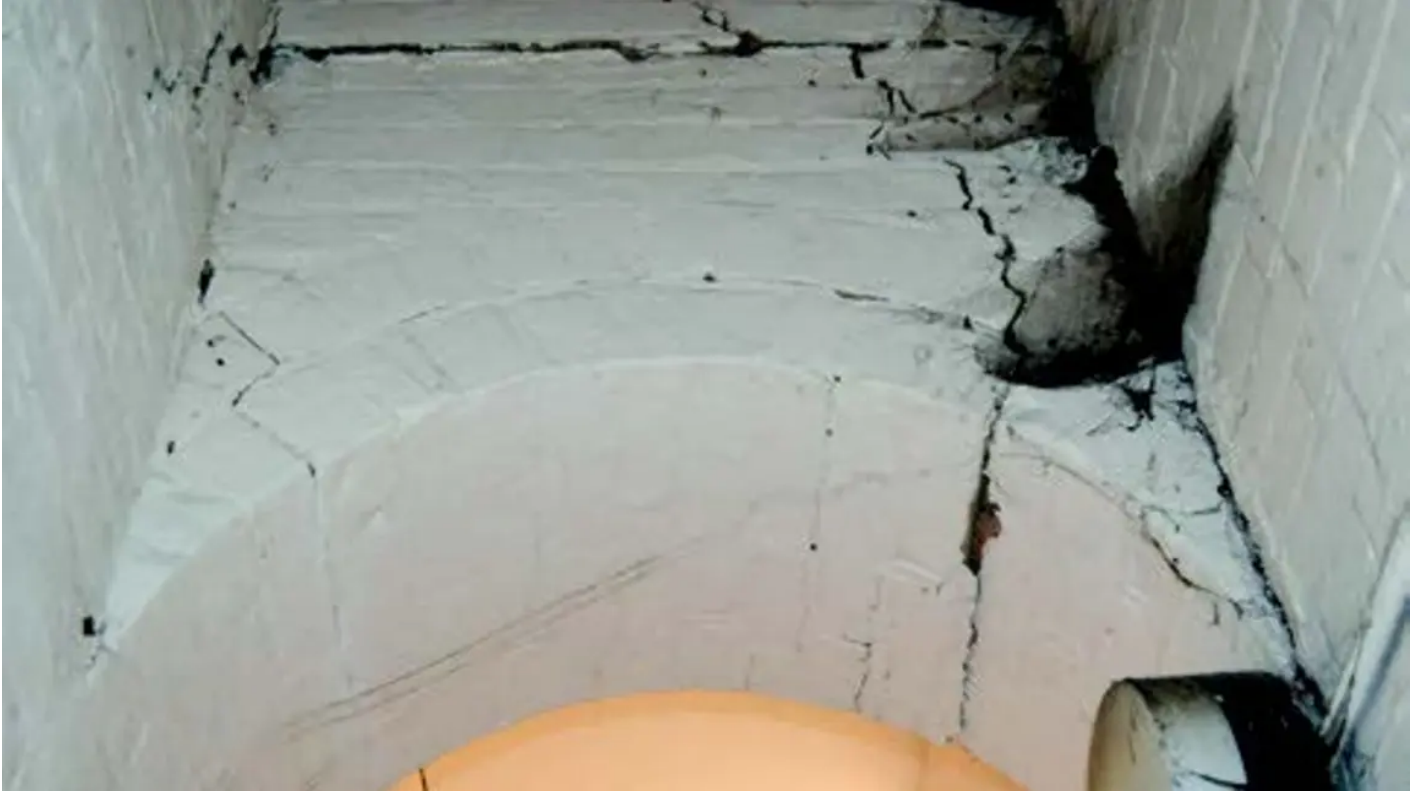
Damage to St Peter-in-the-Forest
