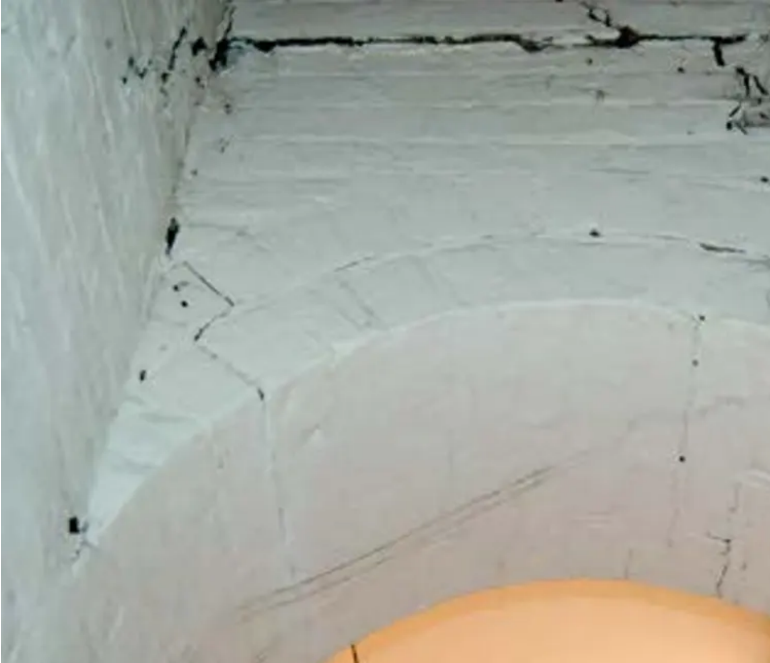
Damage to St Peter-in-the-Forest
