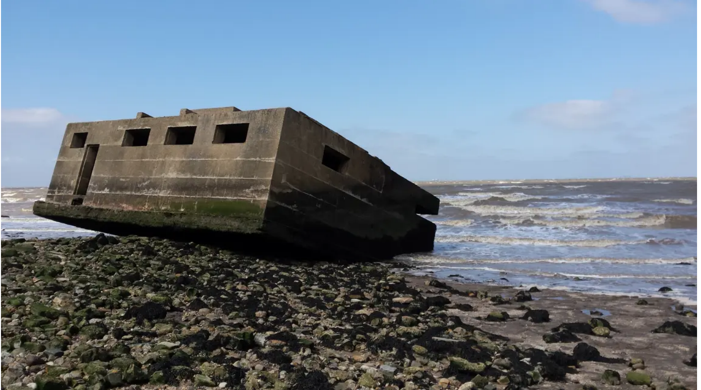
Pill box disappearing in to the sea on the Isle of Sheppey CITiZAN
