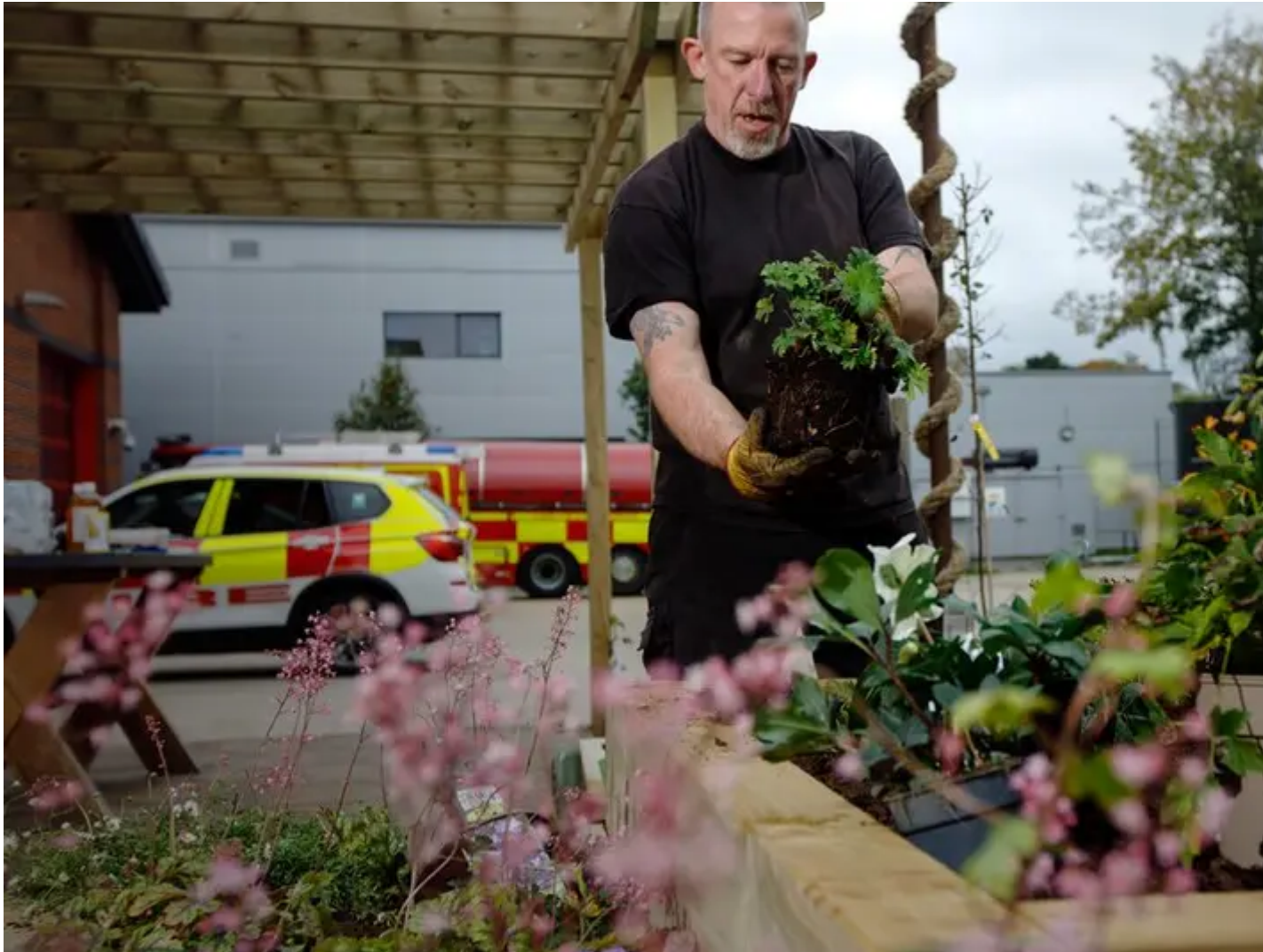
The RHS Communities Team and volunteers build a garden at Guildford Fire Station, Surrey. Photo: Luke MacGregor. Courtesy of RHS Garden Wisley
