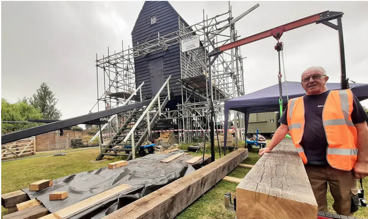
Scaffolding lifted the mill while the huge oak beams that support it were replaced.
