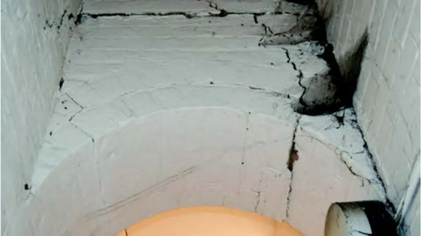
Damage to St Peter-in-the-Forest
